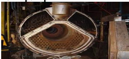
Gambar 2. Bagian filter boiler
